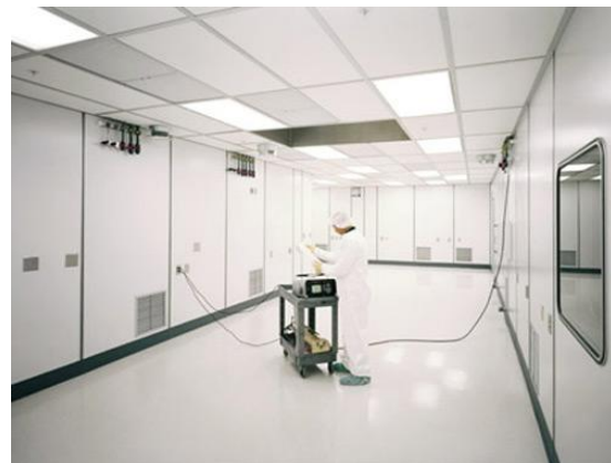
Clean room with piston flow (Shelco Inc).
