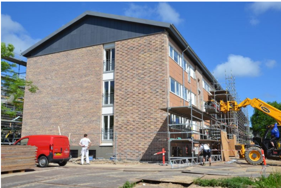
Figure 9. A new brick-wall end facade was erected outside the old end façade built on a new foundation. At the same time new French balconies were installed in the existing end facades. New tiles were attached to the old concrete construction on the entrance façade.
