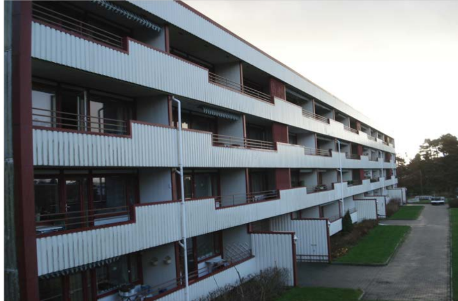
Figure 104. Øvre Kongsgård, Kristiansand. West façade of the case building before refurbishment. Photo: (Kruse Smith).
