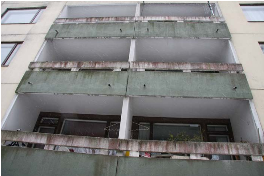
Figure 113. Sahatie 2: balconies in poor condition. Photo: (Pekka Huovila).
