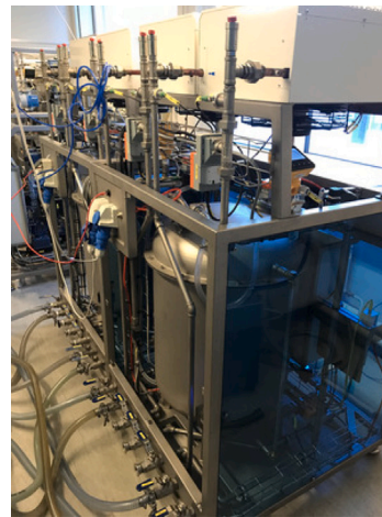
(b) Two consumers, which in total simulate four consumers. The bottom sections are connected to the pipe units. Water then flows up and through the water-to-air heat exchangers at the top, via a control valve.
