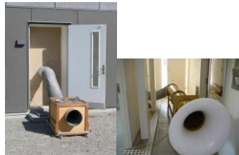
Figure 3. Fan and venturi setup
