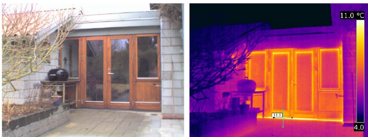
Figure 3. Poorly insulated window/door section along a corridor that connects the main house with an annex.
