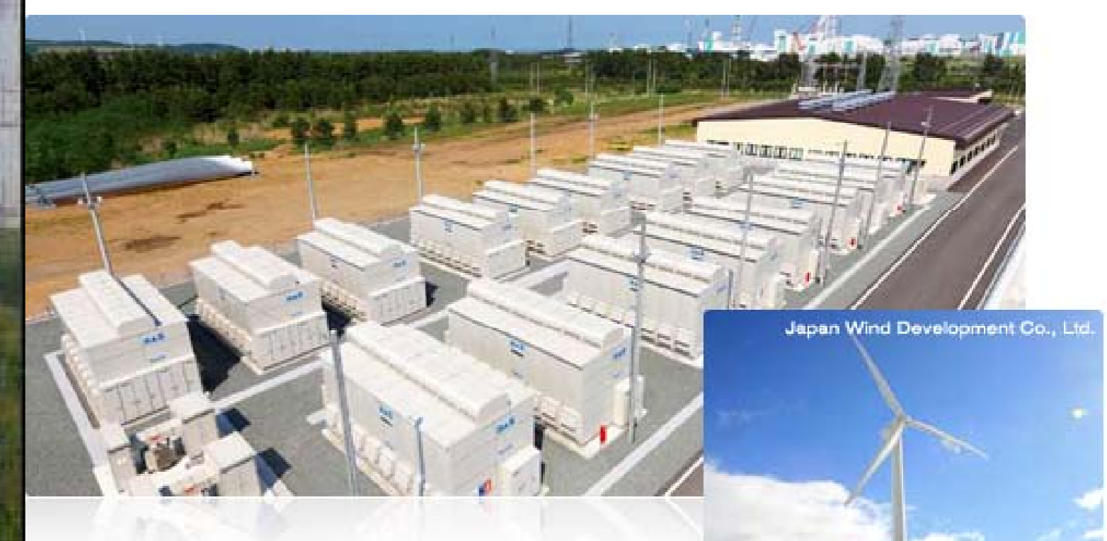
34MW NAS storage, Japan
