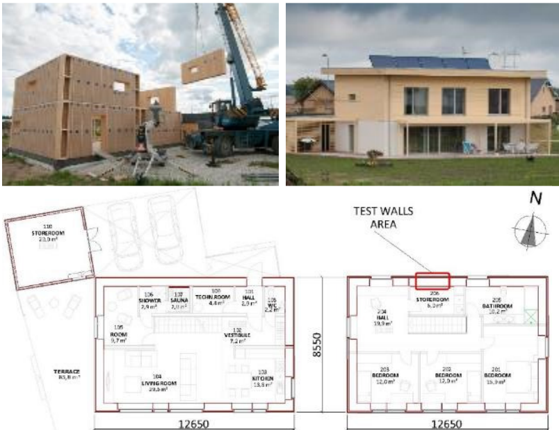
Figure 1. The overall view (above) and plans of the ground (below left) and the upper floor (below right).
