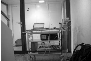
Fig. 9 Infrared-spectroscopy concentration measurement in the pressurized escape stairwell
