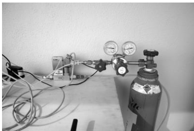
Fig. 6 Dosing equipment with massflow controller and tracer gas bottle (right)
