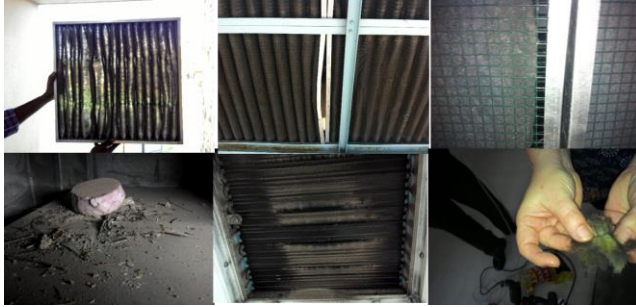
Fig. 3 There were lots of problems with current ventilation system operation and filtration.
