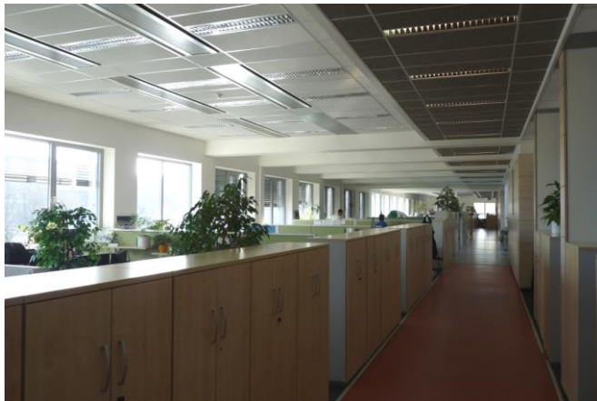
Fig. 1 The view to 4 th floor of open plan-offices and ceiling with chilled beams system
