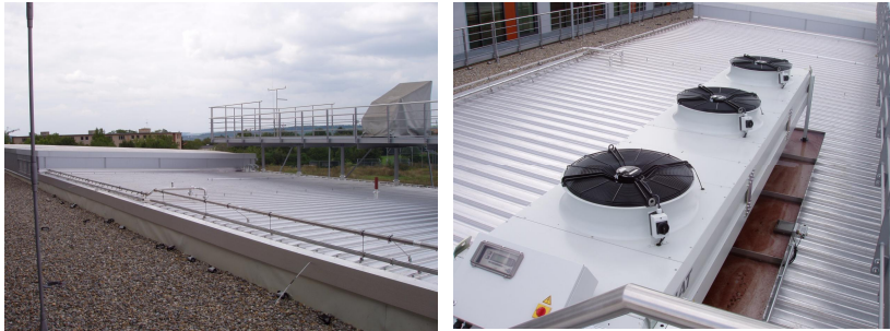
Fig. 2 Passive infrared night cooling fields (left), re-cooling unit and PINC fields (right).
