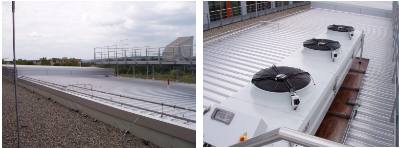
Fig. 2. Passive infrared night cooling fields (left), re-cooling unit and PINC fields (right).
