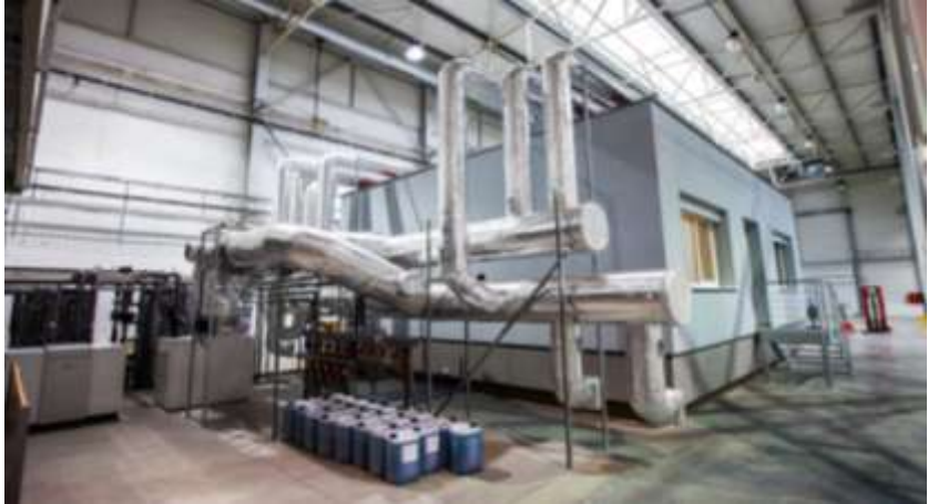
Fig. 3 The consumer model showing the heat pumps for the climate chamber (not-shown) (Photograph by Grul, R.)
