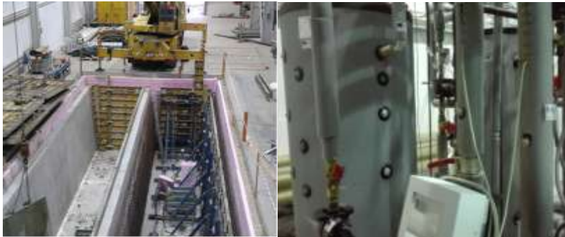
Fig. 2 Left: Insulated long-term heat storage tanks under construction with operating temperature between 15-85 ° C; Right: Short-term heat and coolth stored in 1,000 litre tanks
