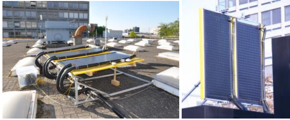
Fig. 1 Installed absorbers on the roof of the Energy Research Lab (right)
