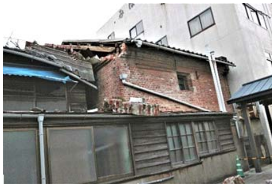
Figure 2: The red brick warehouse right after the earthquake
