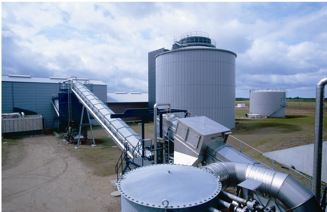
Figure 8: The co-digestion plant for OFMSW and sewage sludge in Grindsted, Denmark (Shredding and conveyor equipment for OFMSW in the front, reactor in the background); (Photo: T. Skøtt)
