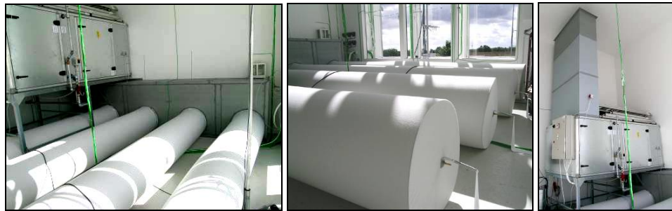
Figure 3-3. KE-low impulse fabric ducts in experiment room (left, centre), Ventilation system in experiment room (right).
