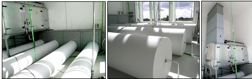
Figure 3-3. KE-low impulse fabric ducts in experiment room (left, centre), Ventilation system in experiment room (right).
