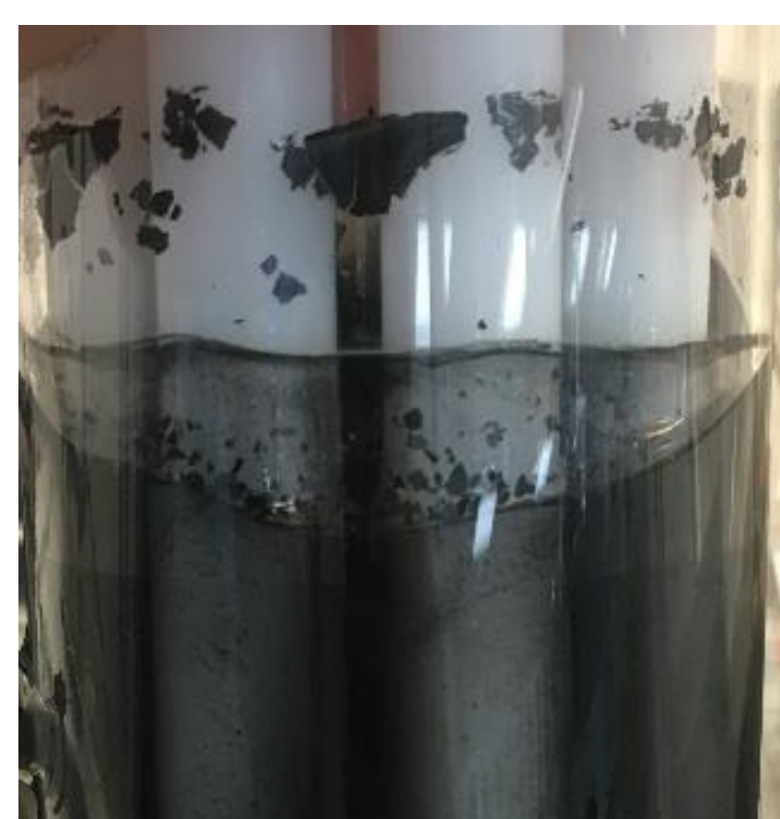
Fig: 3b Corrosion in Pipes
