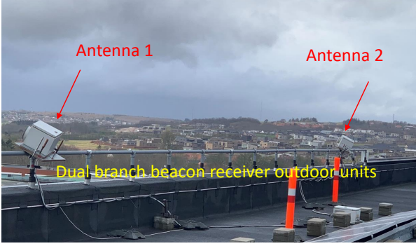
Figure 4. A photo of the dual-branch beacon receiver outdoor units.
