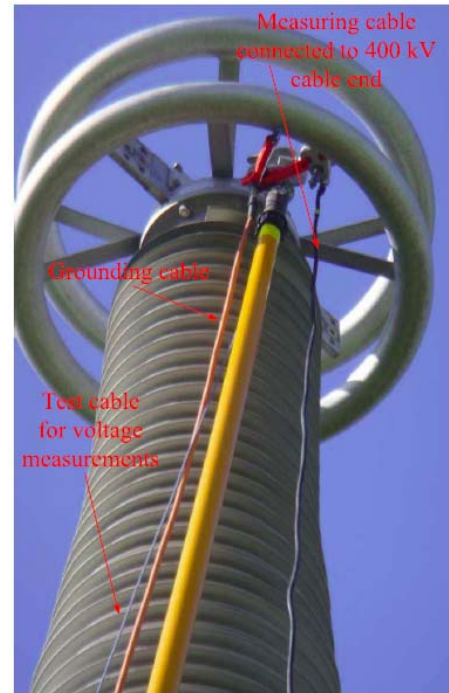
Fig. 9 Measuring and grounding cables connected to HV cable end.
