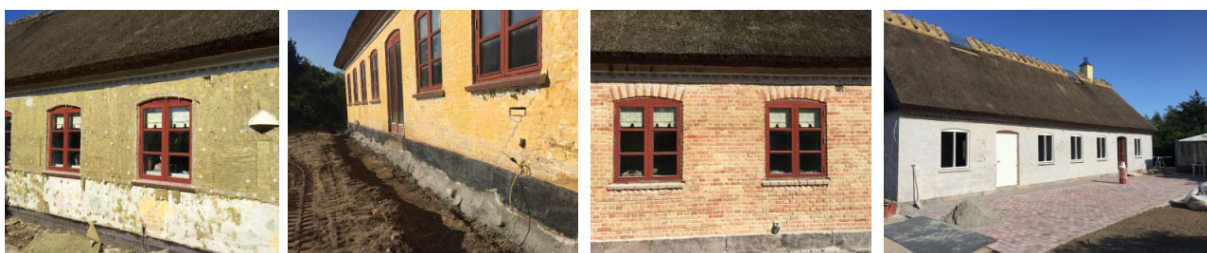
Figure 2. Exterior façade of the building during renovation. Left: exterior insulation removal, mid-left: added protection (sand and concrete) to the foundation, mid-right: cleaned brickwork, right: facade with washed mortar applied. Photos: Thomas Svendsen.
