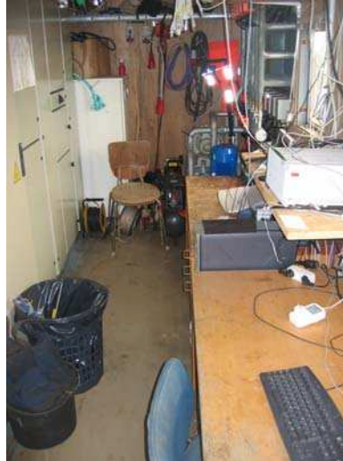
Fig. 6: Inside the control room of Wave Dragon, the PLC and Frequency inverters are in the cabinets to the left, in the far corner the piping, valves and blower for the automatic buoyancy can be seen, and to the right are the SCADA and data acquisition PCs in front of windows looking out onto the reservoir.
