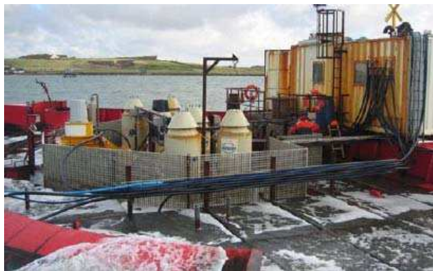
Fig. 12: Trash rack with 5 x 5 cm grid openings enclosing the turbine area.
