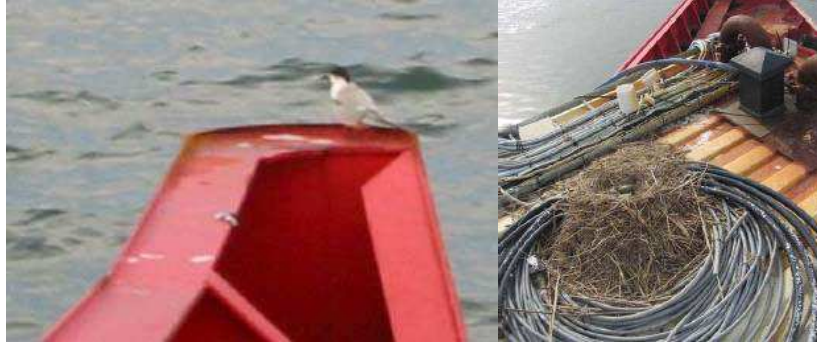
Fig. 4: Bird life in Nissum Bredning. An Arctic Tern perches on the tip of the reflector wing, and a Herring Gull has made its nest in some spare cable on the roof of the control room.
