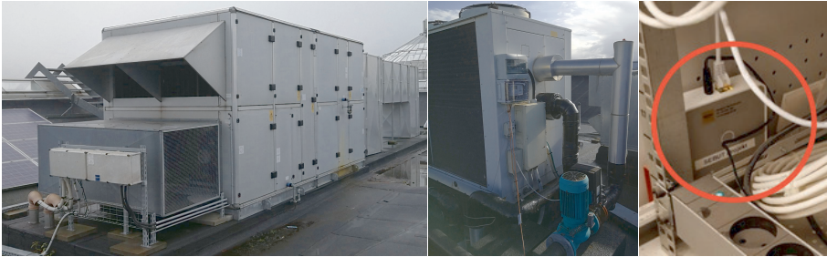
Fig. D.1: From left; AHU, chiller unit and Building Management System (BMS) gateway for remote data acquisition and control, situated at Kolding Storcenter, a Danish shopping center.
