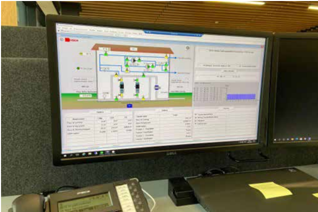
Figure 2. The SCADA system, with a real-time overview over the functioning of a pumping station managed by the water utility of Lemvig (Photo: Jonas Falzarano Jessen)
