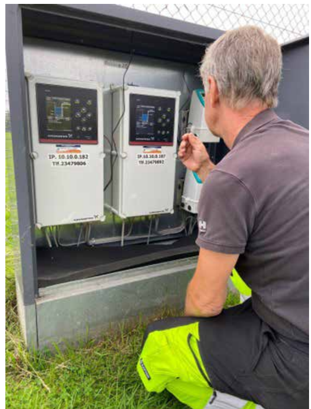
Figure 4. Brad, interacting with one of the physical controlling units supervised by the SCADA system (Photo: Jonas Falzarano Jessen)
