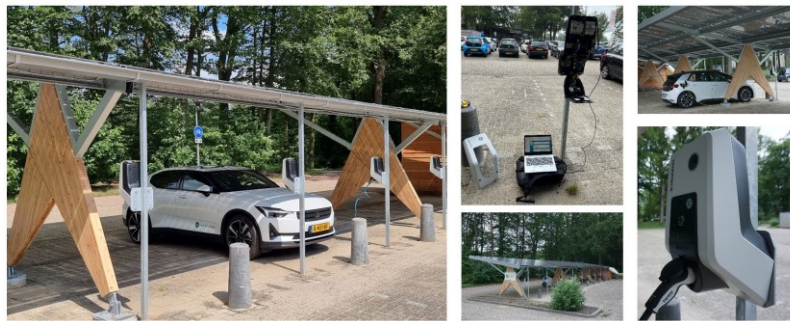
Figure 1. The EV charging station at the UT campus, i.e., SlimPark
