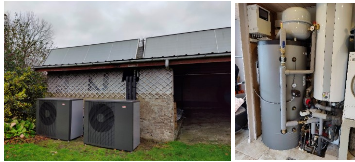
Figure 4. Installed HPs and thermal storage on the Danish demo site
