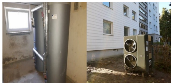
Figure 7. DHW (Domestic Hot Water) tanks and GSJ 46EVI HP in the Polish demonstration site
