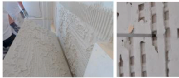
Fig. 14. a) Many insulation products are installed with glue mortar on both insulation and the wall as illustrated. b) The resulting contact can be down to 25 % instead of 100 % contact as given by guidelines [50].
