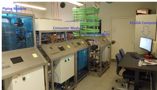
Fig. D.3: Smart water Lab at Aalborg University with SCADA computer at right, pumping and consumer modules visible in the center, and Piping module at left.
