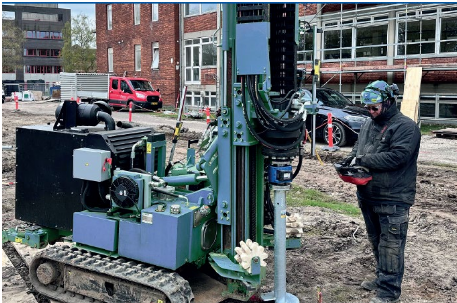
Figure 3-12. Direct method: In-line transducer placed between the torque head and the screw pile being installed.
